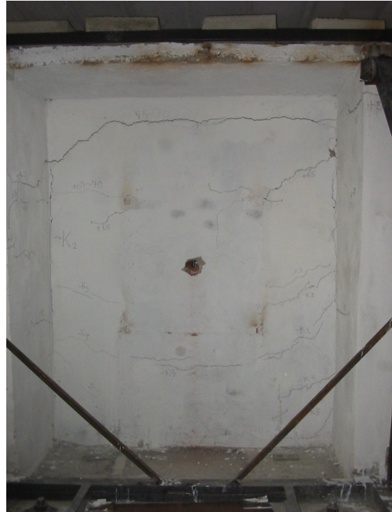
Figure 15. The cracks occurred at the back face of MW under out of plane cycling load.
